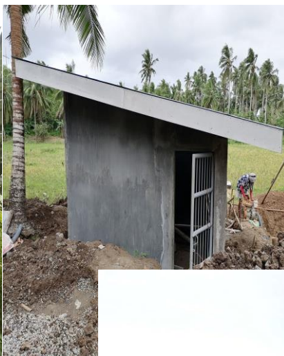
Solar Panel & Pump House of Main Canal 2, MACALELON SRIP
