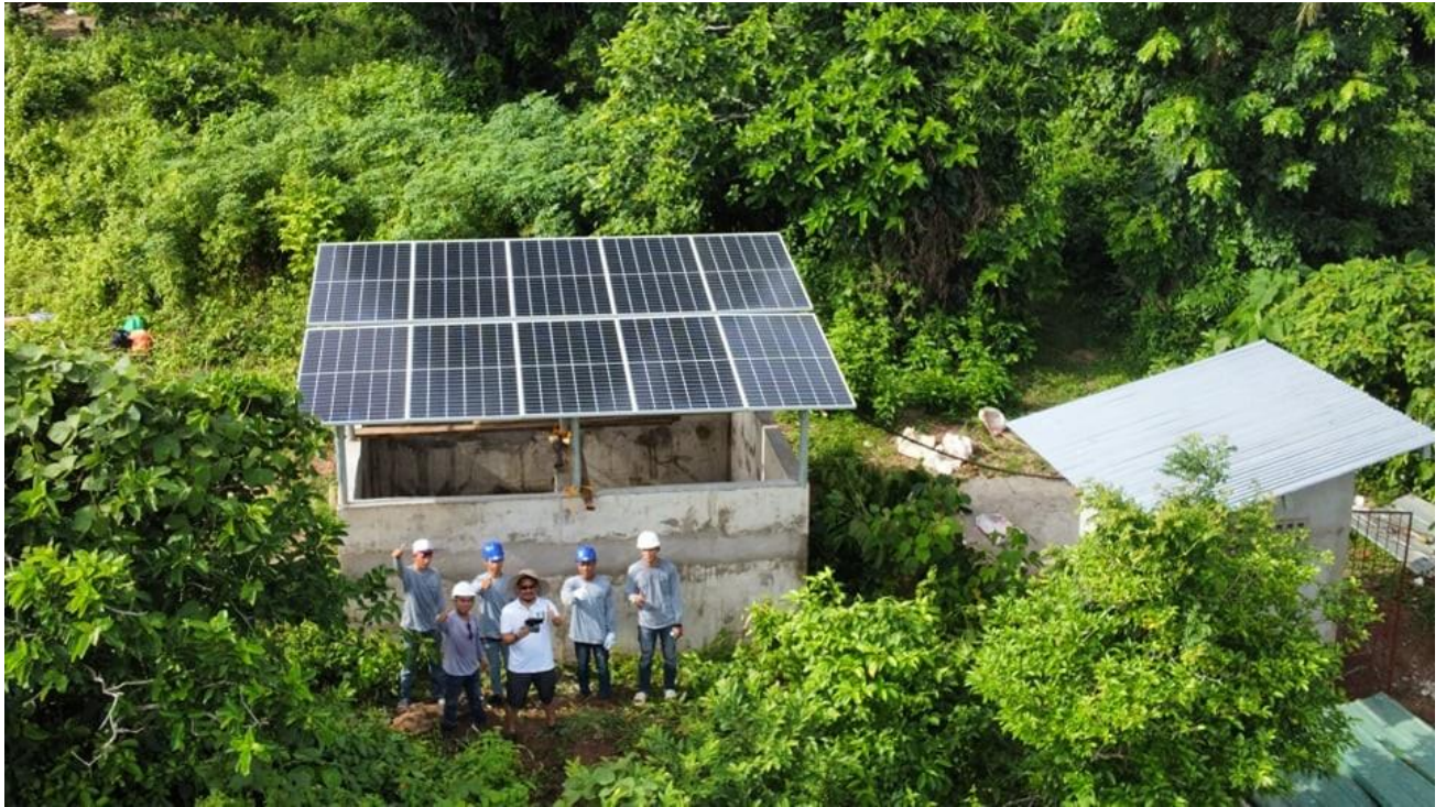
Completed Solar Powered Project, Talisoy SIP in Region 4A
