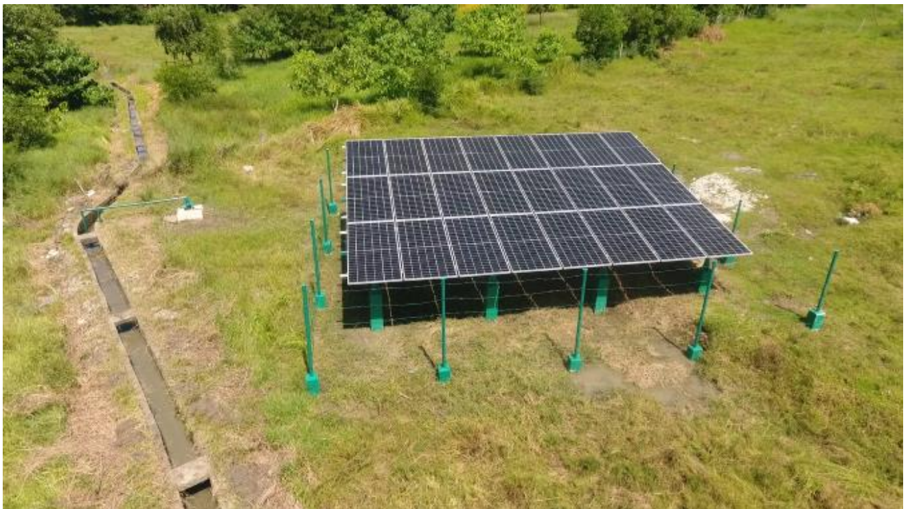
Completed Solar Powered Project, Llano PCIS in Region 4A
