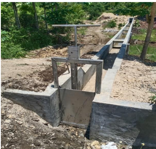
Irrigation Facilities, BONOT-BONOT SRIP
