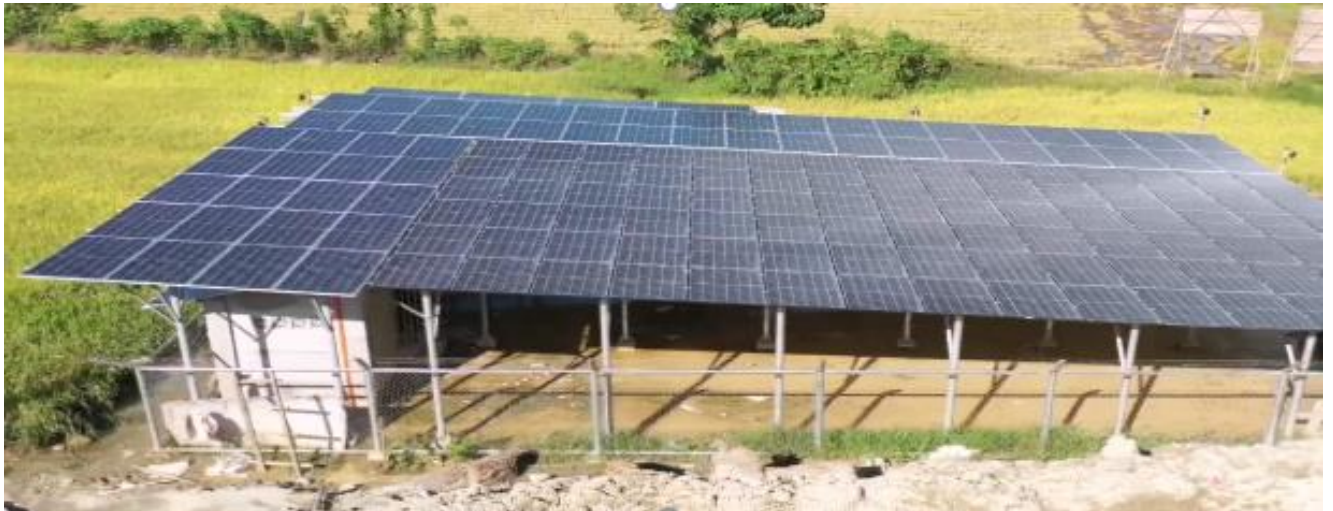
Solar Powered Irrigation Pumps
