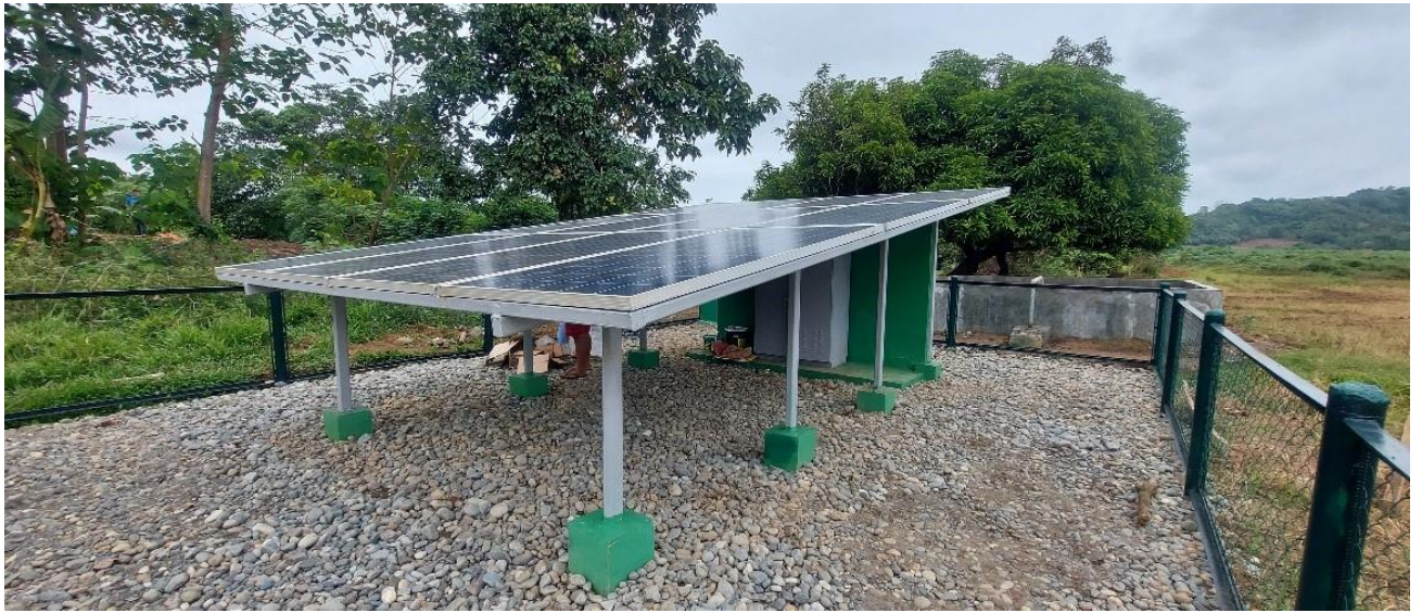
Completed Solar Powered Project, Sta. Isabel PIP in Region 2
