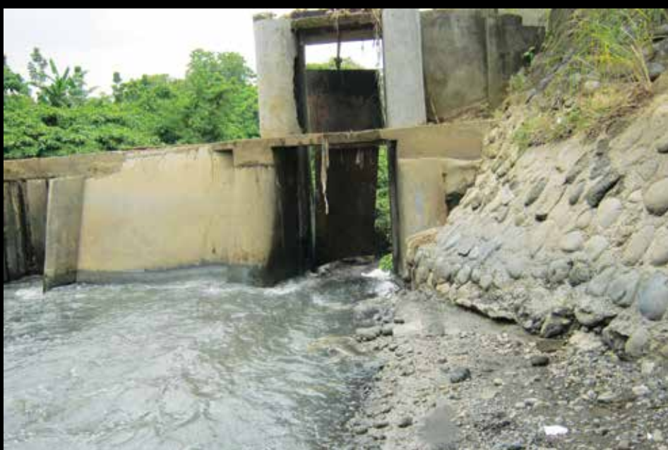
San Cristobal River Irrigation System Brgy. San Cristobal, Calamba Laguna
