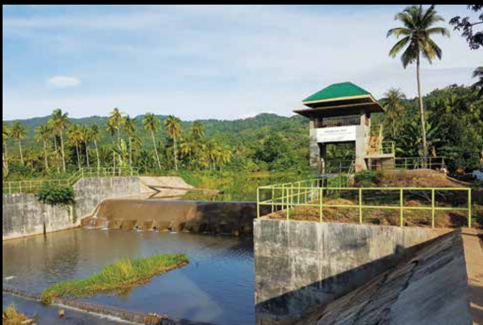
Baleguian Communal Irrigation System Jabonga, Agusan del Norte
